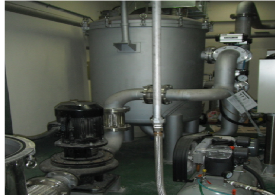
Filtration system (Busan station)
