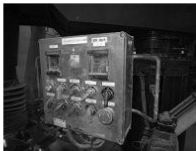
<damper control panel>
