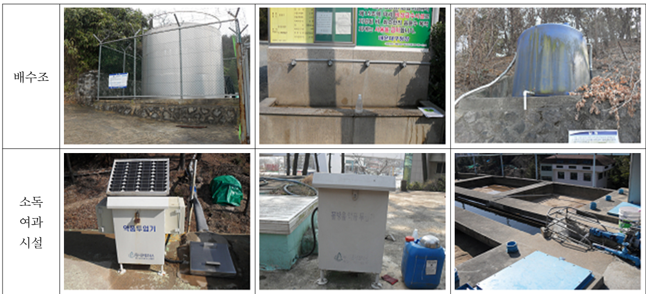
Fig. 2. Drainage tanks and disinfection filtering facilities in small-scale waterworks.
